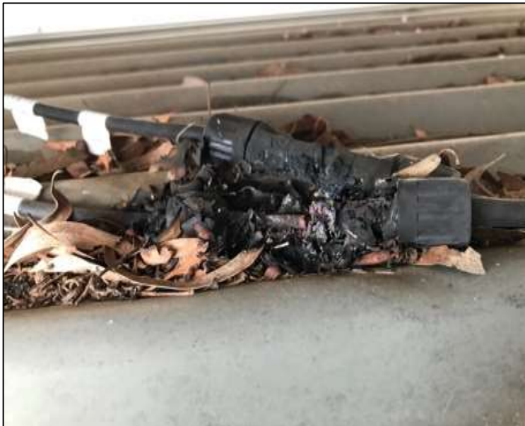
Charred leaves and windblown material under a solar panel
